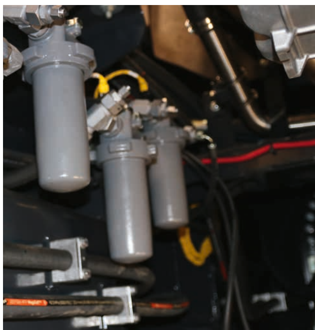
Hydraulic filter system.
